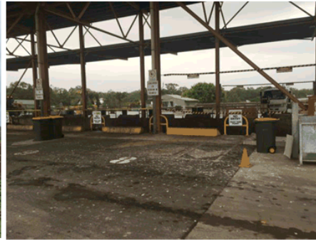
Figure 4 Evidence of bird activity at Bundaberg transfer station.
