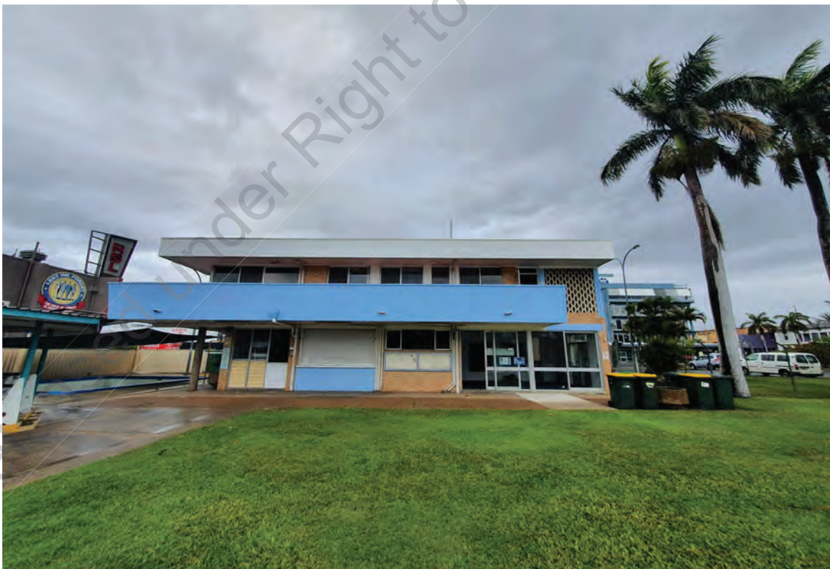
Figure 4: Northern elevation of Entrance Building/Caretaker's Residence (1971) from within the pool grounds (Queensland Government, 2022)
