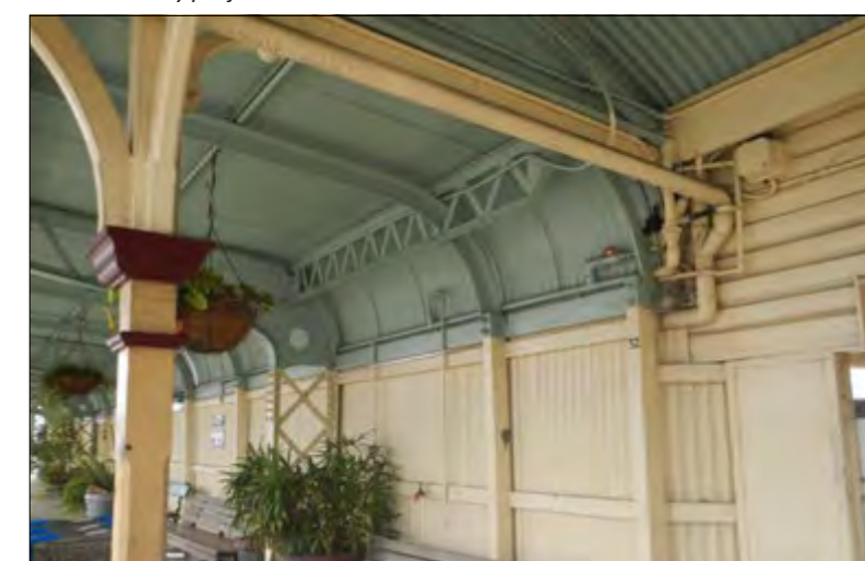
Detail of western platform extension illustrating change in building style and material.
