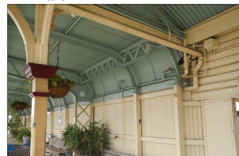
Detail of western platform extension illustrating change in building style and material.
