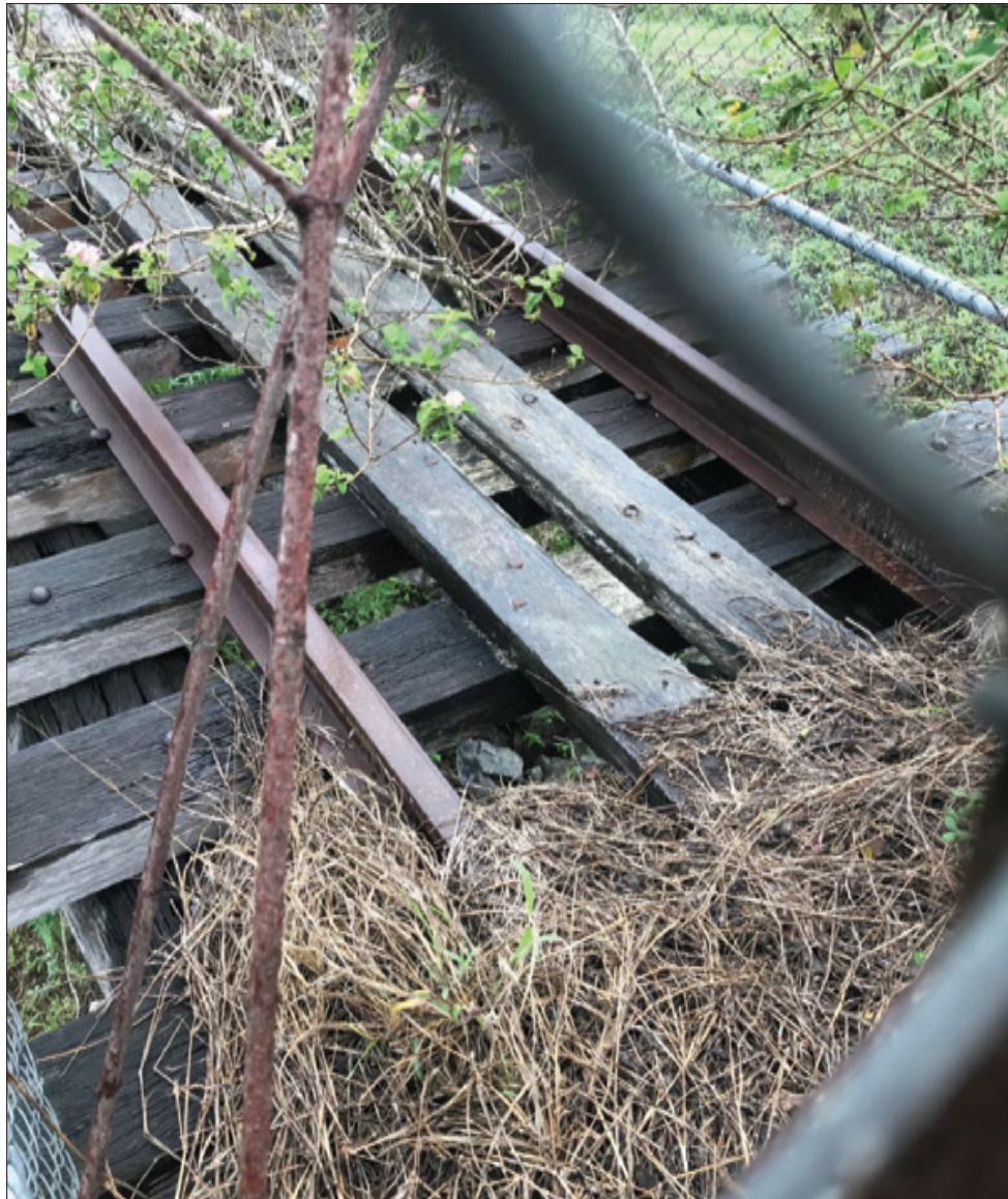
Figure 2-4: Close-up view of the transoms and the condition of the girders from the top.
