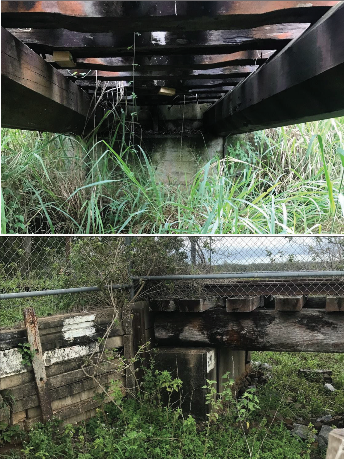
Figure 2-5: View of both abutments, Abutment 1 on top and Abutment 2 the bottom image. Both abutments are concrete piers with the wingwalls consisting of concrete panels held in place by sections of the steel railway line. This is a typical abutment configuration for this period of railway construction and is a testament to the original construction and should be retained as they are in fair condition.
