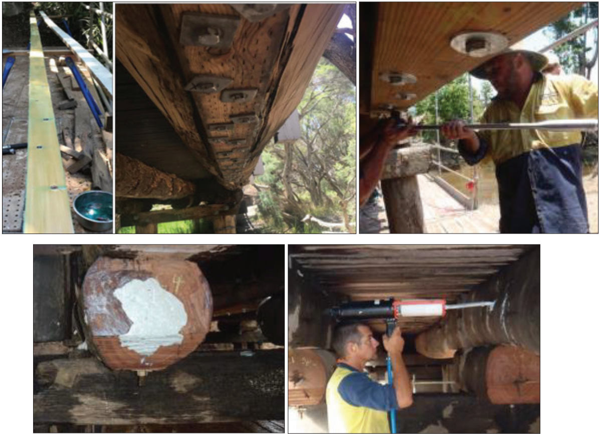
Figure 6-5: The repair of Meachams Bridge in Cassowary Coast. The bridge was retrofitted with fibre reinforcement on the bottom of the girders, some corbels and girders were injected with a high strength epoxy. Some piles were also wrapped with high strength fibre and injected with epoxy, then the entire bridge was diffused with borate salt rods to neutralize decay growth.
