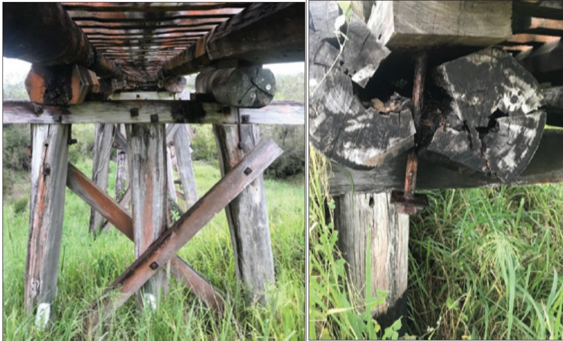
Figure 2-9: View of one of the pile bents on approach 1 side of the creek. This bent consist of three driven piles and overall in fair condition. Most of the corbels in these bents are in fair condition, however there was only one corbel found that had crushed and failed due to the vertical through bolt allowing moisture in which lead to the member decaying.
