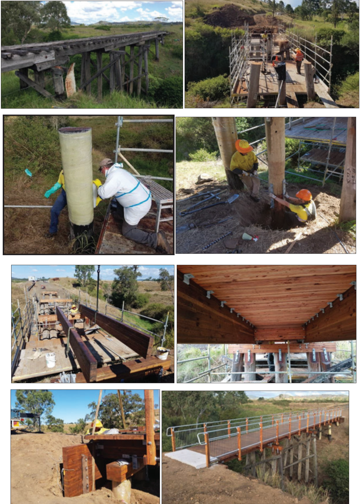
Figure 6-4: The photo series above demonstrates Option 3 type of fix that was done for Jimmy Gully Bridge along the BVRT. The existing poor condition superstructure was removed and the piles were repaired with high strength fibre or posted with new section. New glulam back wall, caps, girders and deck system was installed utilising a horizontal connection detail.
