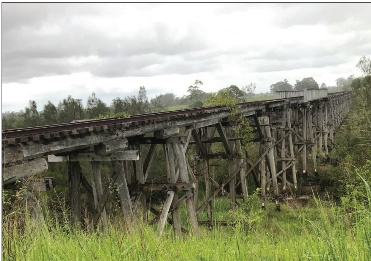
Figure 2-1: View of Splitters Creek Bridge from end 1. There is 7 timber approach spans on Side 1 (Eastern Side) of the creek which is spanned by 2 continuous steel through plate girders supported by a centre timber bent (trestle) in the creek. There is a large amount of vegetation growth around the timber bents which keeps the moisture content high in the timber. When the moisture level in the timber is above 22%, decay-causing fungi can start to grow; when the moisture content drops below this level, the fungi become dormant and decay will be arrested until the moisture content rises again.
