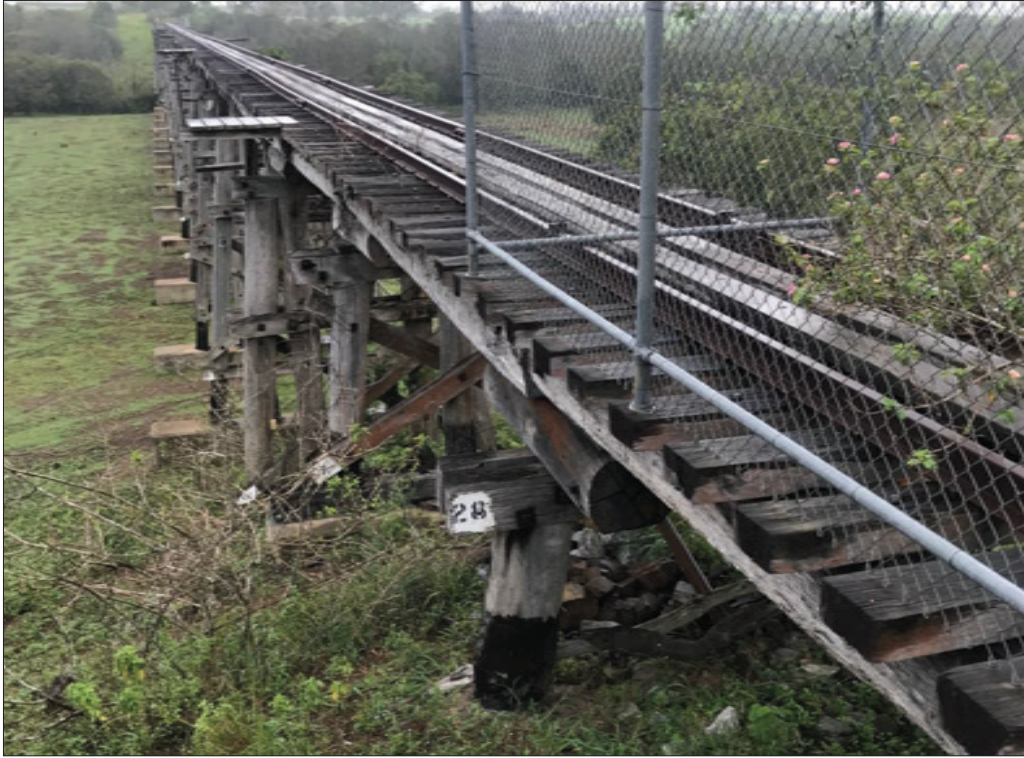
Figure 2-2: View of Splitters Creek Bridge from end 2. There is 18 timber approach spans on Side 2 (Western Side) of the creek. Unlike side 1, the vegetation is quite low and clear under and around the bridge as cattle continually graze this area. Note Bent 1 consists of driven timber piles (Pile Bent), while the remaining bents of this side are constructed from timber posts bearing directly on a concrete footing (Frame Bent). Note the fence to prevent pedestrian or vehicle traffic.
