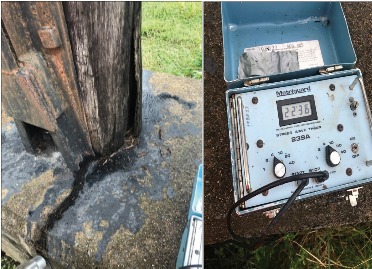
Figure 2-11: As described above, the bottom sections of the timber posts were determined to be a ‘hotspot’ for decay and determined to be an ideal area to test using non-destructive methods, such as EPHOD® Stress Wave Technology. Refer to Appendix A for more information of this type of testing method. The reading of 2236 \mu s recorded is the time taken for the compression wave to travel across the section of the member tested. This was recorded at the bottom of one of the posts and was found to be similar across 25% of the posts. Deterioration of this magnitude means that the Modulus of Elasticity/Modulus of Rupture in various stress directions (wood is anisotropic with different strength properties in different directions) has deteriorated to an extent that the element can no longer support its own dead weight. Readings between 1000 \mu s and 2200 \mu s indicate that the member cannot carry its own dead weight in these regions. Readings in excess of 2200 \mu s can signify a cavity while a reading above 3300 \mu s indicates the element can no longer support its own dead load and is at risk of failing at any point. It can also be noted that roughly 1m above the concrete footing the post had readings around 600 \mu s which signifies sound (solid) wood resulting in only the bottom portions requiring require. It is highly recommended to conduct a detailed inspection of the entire substructure utilizing non-destructive technology through the use of the Stress Wave Timer (SWT) machine. Also note that termites were found at this particular location and it’s unknown how many other areas of the structure are affected. It is estimated that 25% of the posts will require repair at the bottom 1m section of the post and 10% will require full repair/replacement. Refer to Section 5 for a full list of recommended repair options for refurbishment to a pedestrian/cycle bridge.
