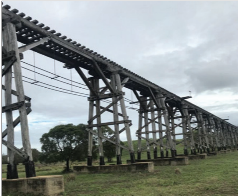
Figure 2-6: An overall view of the timber approach spans of side 2 from the creek bed. The 11m long girders are supported by struts (knee braces) attached to the frame bents which effectively reduces the span length and helps transfer the load from the superstructure (girders) into the substructure (posts). This allows smaller (more accessible at the time) girders to span a longer length and keep the number of bents down as they would have been a large percentage of the overall cost of the bridge. The girders bear directly on corbels which sit on the headstocks. The headstocks transfer the load into the 4 posts (some posts have 5 posts) and down into the concrete spread footing. The timber sashes (horizontal braces) and cross bracing provides lateral support for the tall bents. The full length shoes for the knee brace attachment to the girders is an interesting design not typical of the period.
