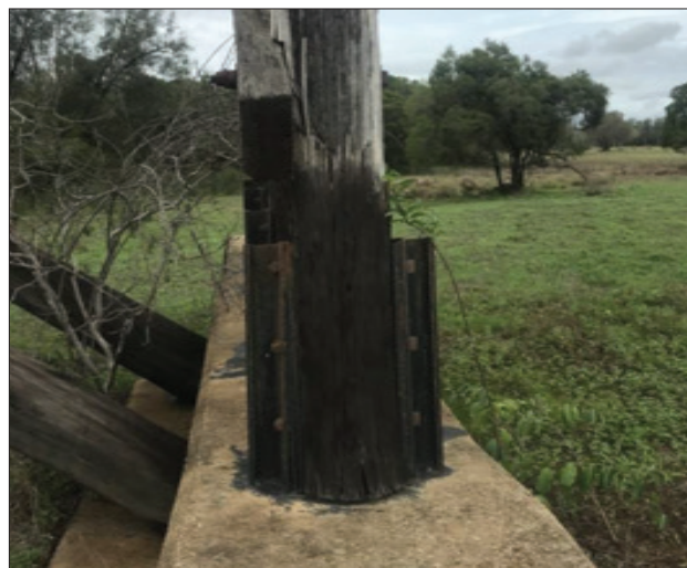
Figure 2-10: The typical detail of the post hold down connection is two large steel plates (railway line) embedded into the concrete footing that connects to the timber post with 6 horizontal bolts. As shown in Figures 2-11 & 2-12 below, the bottom section of several posts have moderately to severely undergone decay. This is as per expected due to the timber posts bearing directly on the concrete footing which typically has a high moisture content. Over time the timber post undergoes capillary action and draws up the moisture like a ‘straw’. Once the moisture content in the timber elements reaches 22%, decay causing fungi are activated and the decay process begins. The heavy solids coating on the column bottoms has further increased the moisture retention problem by preventing the element from breathing and reaching equilibrium moisture contents below the point at with decay begins and proceeds (22%).
