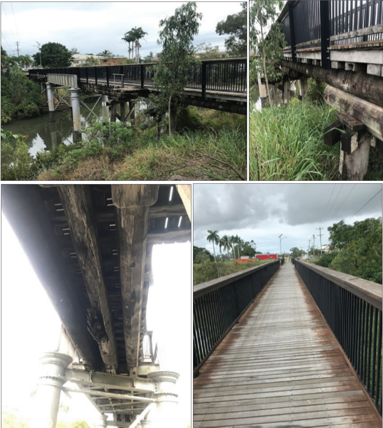
Figure 6-2: The above photo series demonstrates an Option 1 type of refurbishment (build off existing railway bridge) used for the construction of a pedestrian bridge along the same railway line as Splitters Creek Bridge and is located just off Quay Street on the North-East outskirts of Bundaberg CDB. The existing railway bridge was left un-touched and a new hardwood deck system with handrails was installed. Six 100mm x 250mm timber joists were placed on top of the existing transoms (rail ties) with a 38-50mm thick hardwood deck installed on top. This option will likely be the lowest cost but also carries the shortest expected lifespan. As seen in the bottom left photo above, one of the girders has failed and fallen out creating a ‘weak’ point along the bridge. Due to a high residual capacity of timber and the continuous joists, a complete failure of the bridge (span) hasn’t occurred yet but is only a matter of time unless extensive maintenance is undertaken.
