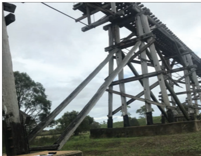
Figure 2-7: Several of the bents have log longitudinal bracing that extends from the concrete base of one bent to the top sash of the bent being supported. This bracing is repeated on the other side of the bent. This type of stability repair is seen in two other locations along the bridge.
