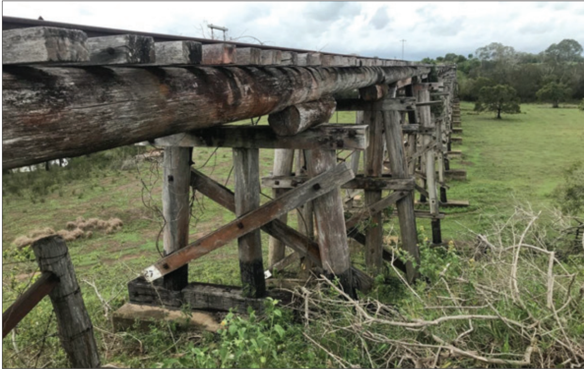
Figure 2-13: The girders and corbels of the two lower spans at Abutment 2 end was also briefly tested with the SWT machine. The adjusted values of most of the readings did not exceed 700 microseconds. This suggests that the timber at the locations tested is still in fair condition and will be suitable for use in carrying pedestrian loadings. However this is only a small sample size and it is highly recommended to conduct a detailed inspection of the entire superstructure using of the SWT machine. As mentioned previously the vertical fasteners that connect these members together increase the rate of decay in timber as they allow moisture to travel down the fastener into the heartwood of the girders and corbels, therefore increasing the moisture content in the middle of these elements. The heartwood of a log element is less capable of breathing and expelling moisture than the sapwood that surrounds it, so vertical connectors funnel the moisture directly into the heartwood accelerating decay. Once the moisture content exceeds 22%, timber consuming fungi are activated and the decay process begins. It is estimated that 10% of the corbels and girders will require repair/replacement. Refer to Section 5 for a full list of recommended repair options for refurbishment to a pedestrian/cycle bridge.
