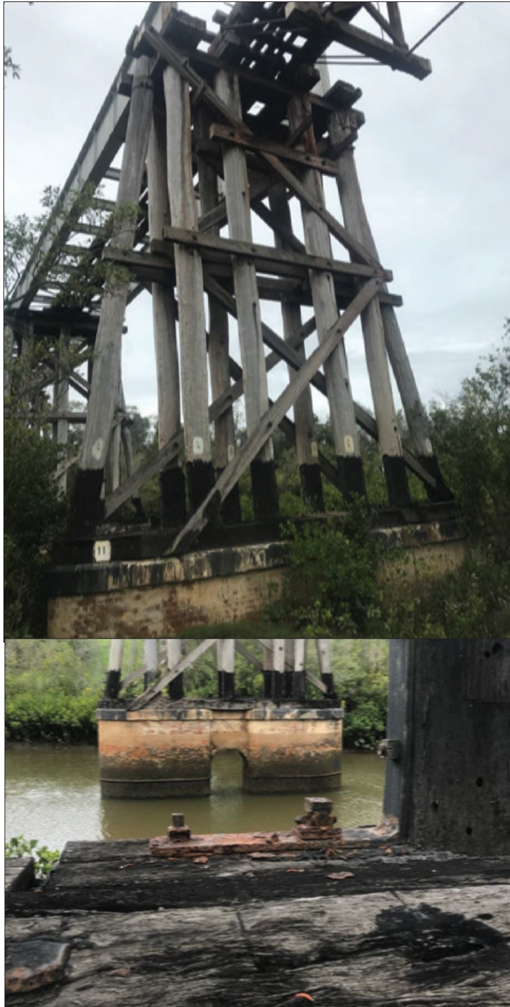
Figure 2-8: There are three larger timber frame bents that support the two steel plated girder spans over Splitters Creek. These bents consist of 12 timber posts that bear on timber cap wales that help distribute the load into the concrete footings. Overall these bents are visually in fair condition and are very significant to the heritage of the structure. Note the black coal tar coating applied to the bottoms of the columns. This coal tar paint holds the moisture into the bottoms of the columns and the moisture absorbed from the concrete below is not able to evaporate. This is an old method of heavy timber bridge construction that actually shorted the timber component life. Diffusing these areas would be important to preserve and extend the life of the element.
