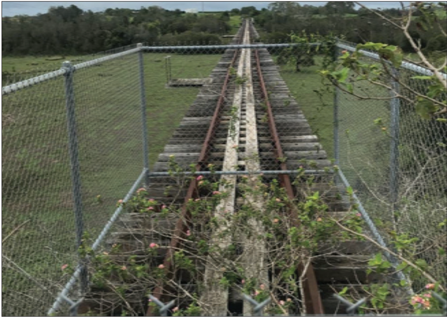
Figure 2-3: View on top of the bridge from Abutment 2. The transoms (rail ties) remain intact along with the railway line and the existing features such as the emergency bays (absent of hand rails on two sides in each case) off the side of the bridge.
